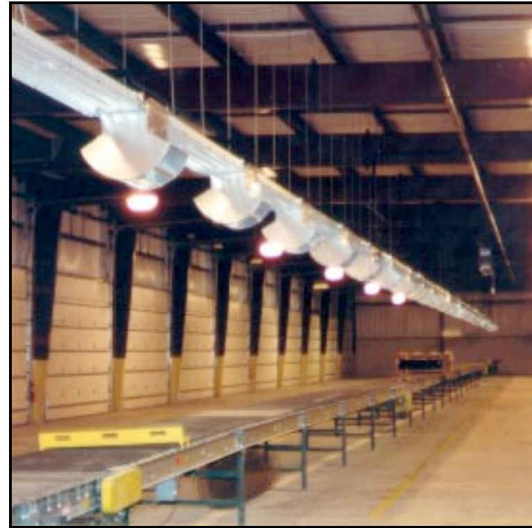
HotZone conveyor heaters directly over, and directing their heat to either side of a freight sorting conveyor
