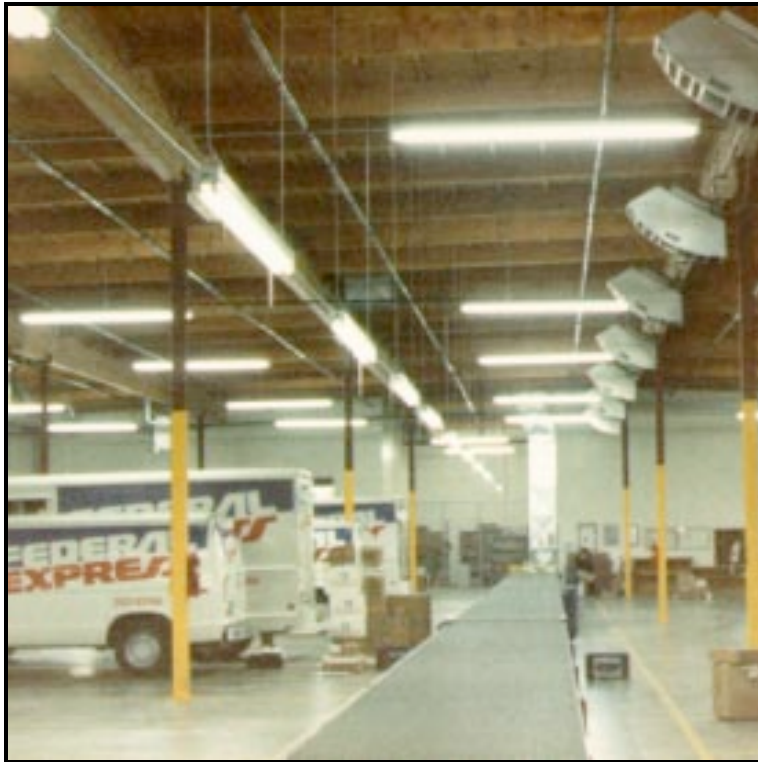
Natural gas HotZone™ aisle heaters directed at the sorting conveyor at an air freight terminal
