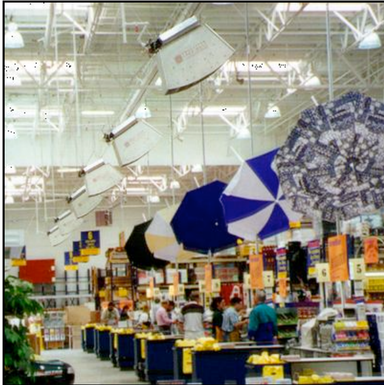
35mBTU natural gas HotZone™ aisle heaters warming the checkout aisles of a grocery store
