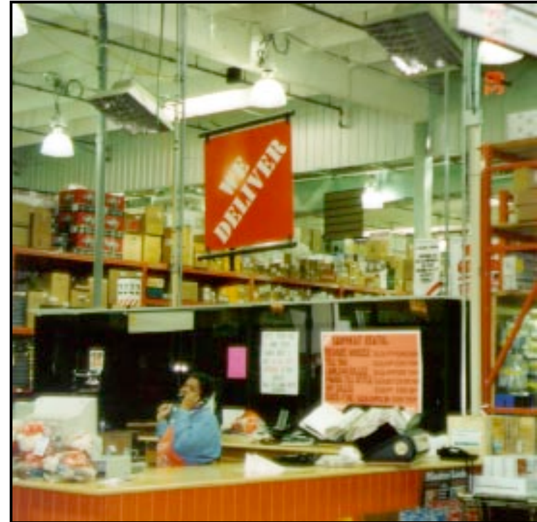
70mBTU natural gas HotZone™ spot heaters warming the customer service area of a home improvement warehouse store
