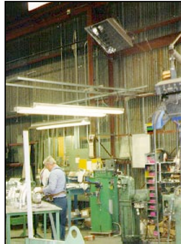
A natural gas HotZone™ heater mounted out of the way of equipment and people spot heating a work station
