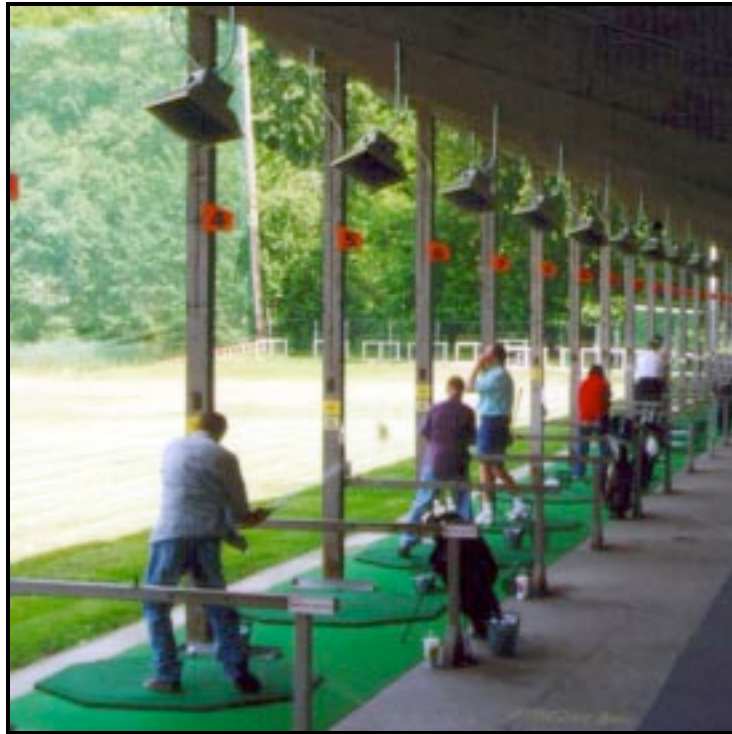
Individually controlled 3KW electric HotZone™ spot heaters extending the practice season at a driving range.
