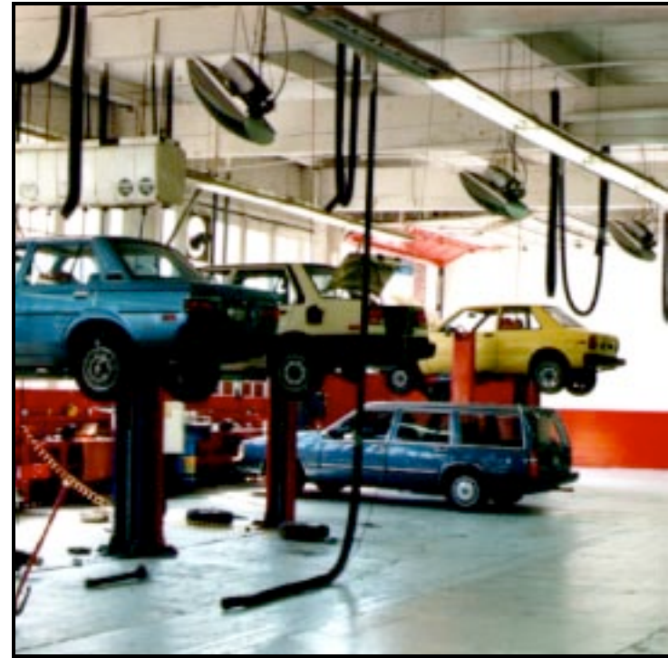
High power electric HotZone™ spot heaters warming people and objects, not the air at an auto repair shop.
