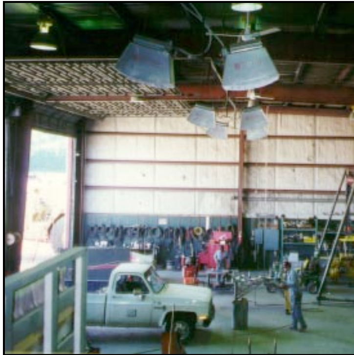
Ceiling mounted natural gas HotZone™ aisle heaters keeping mechanics warm, despite high air exchange.
